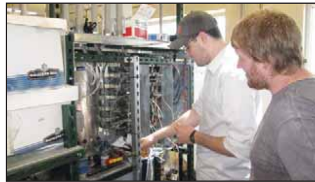
(L to R) Jonathan Warner and Chance Rieger working on data acquisition and control wiring for the triple effect evaporator in the Unit Operations Laboratory. This is a newly designed data acquisition and control system for the remodeled evaporator laboratory experiment. Senior chemical engineering students will use this system for gathering laboratory data and controlling the operation of the triple effect during the CBE 461 Mass Transfer Laboratory in fall 2011.
