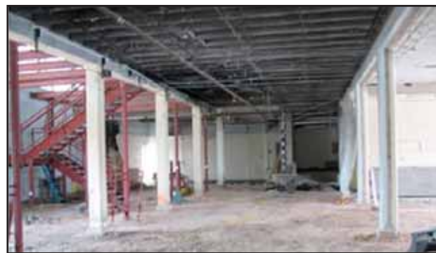
First floor of Unit Operations Laboratory under reconstruction, with central stairway installed.
